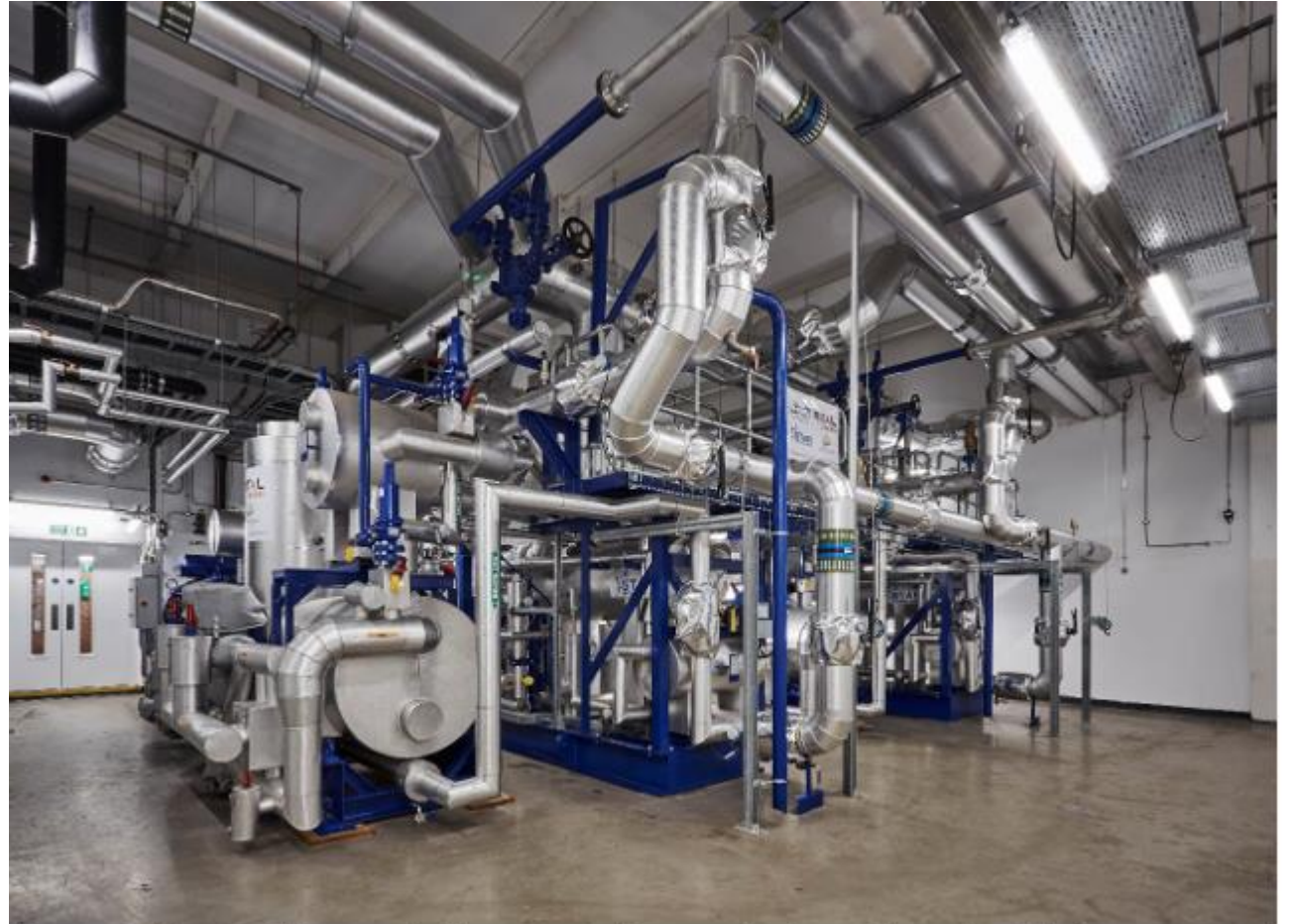
Figure 3: Photo of Ammonia heat pump harvesting heat from the Clyde estuary
